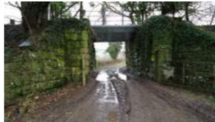
Existing bridge. Path to be shared by all as it narrows to cross the track. Railings to be modified to protect users
