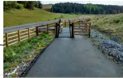
Route to connect with existing path constructed as part of the A465 dualling program
