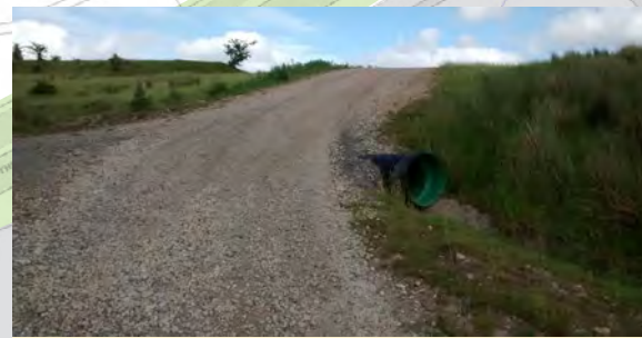
Short steep section to be graded out to improve gradient during surface upgrade
